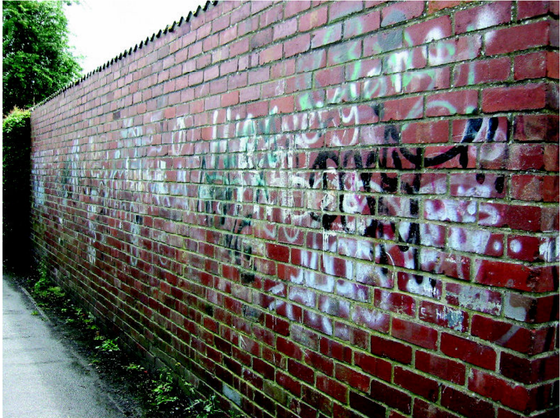
Fig. 3: Graffiti along the wall of the snicket (rear shed wall of 81 Beckfield Lane)
